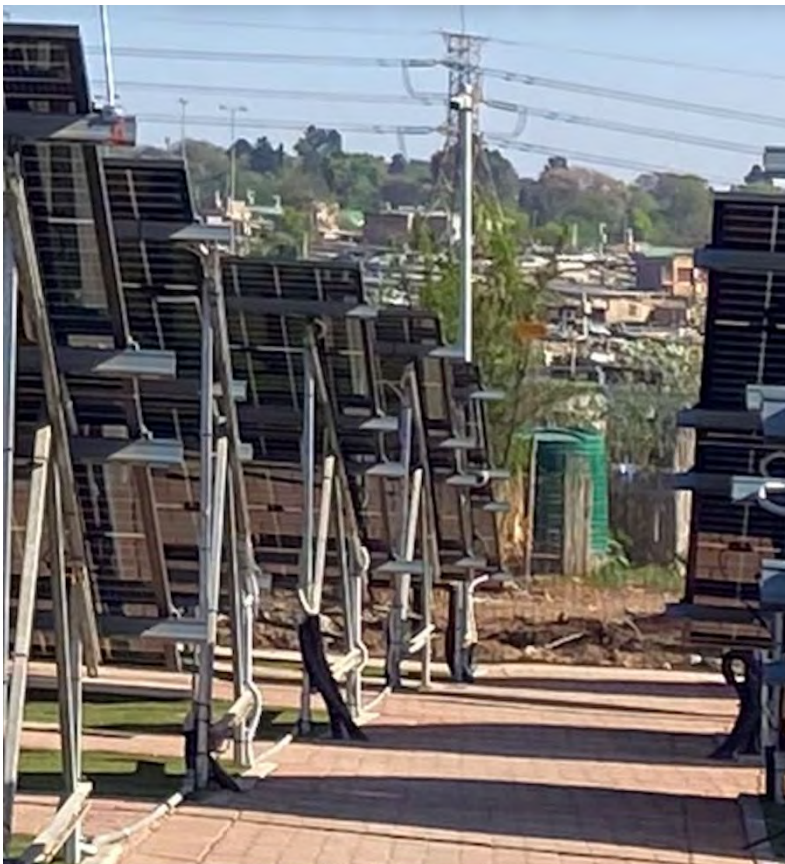
The contrast between old and new, rich and poor, development and underdevelopment: A solar mini grid in Johannesburg adjacent to a housing settlement.
