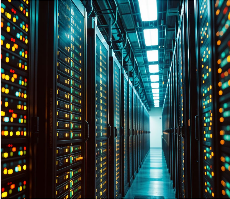
Data centres constantly and rapidly processing incoming information. Photo: Shutterstock
