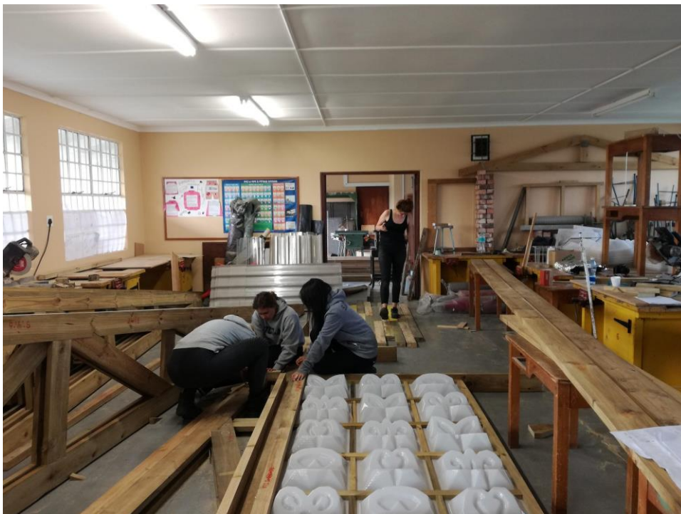
Figure 12: Students make building components in the nearby secondary school workshop. Photograph by author.
