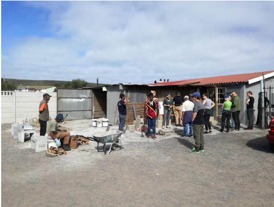
Figure 13: Masonry work completed by students and members of the community. Photograph by author.
