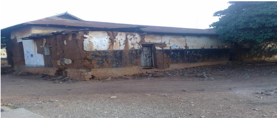
Figure 4. Rundown accommodation occupied by parents and left-behind household members of a migrant.
